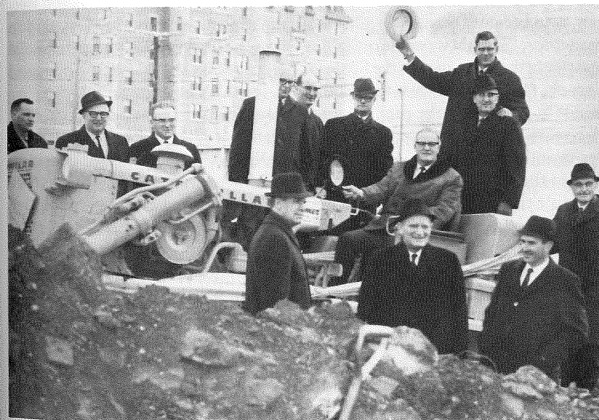
FCL's board of directors celebrate the start of construction of the new head-office building in 1969. President R. H. (Bob) Boyes is driving the bulldozer. Waving his hat in the background is Boyes's successor as president, Gordon M. Sinclair.
